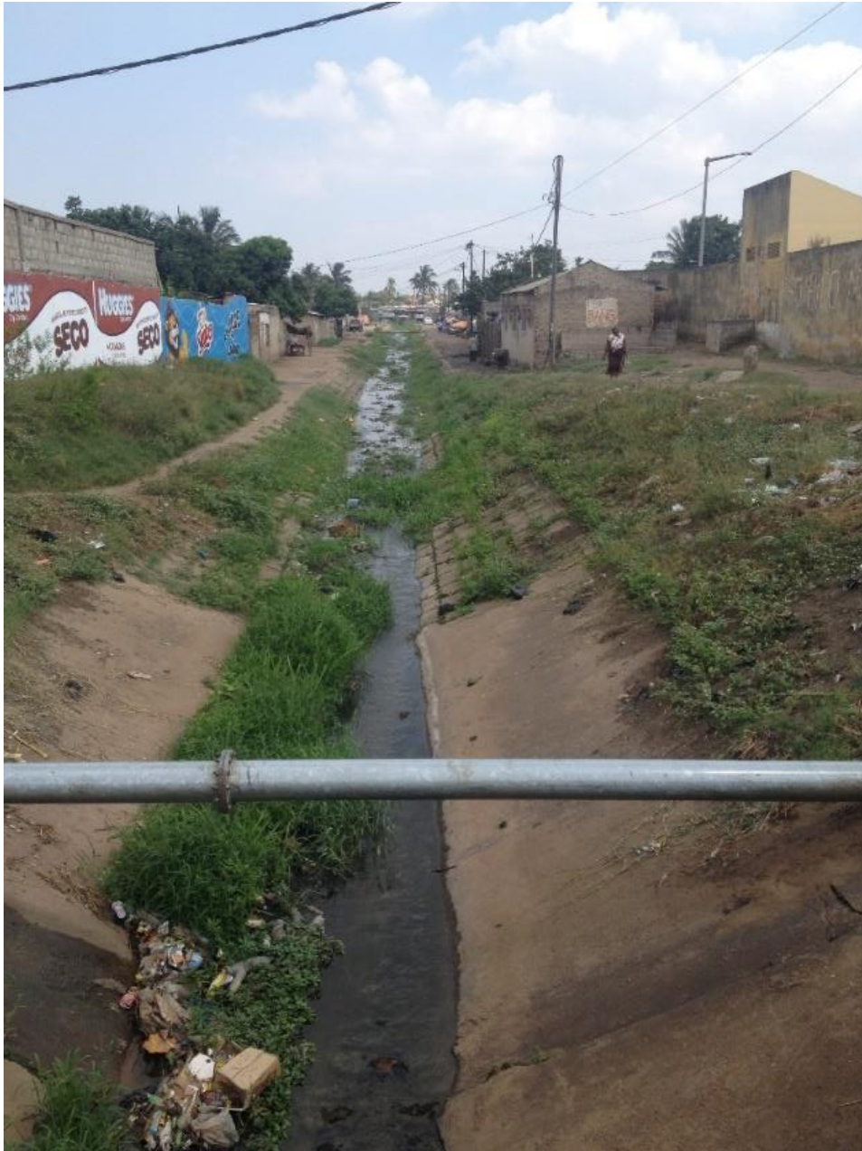
Figure 8: Storm water drainage in the Xipamanine neighbourhood, photo taken by the author 21 st of March 2015.
