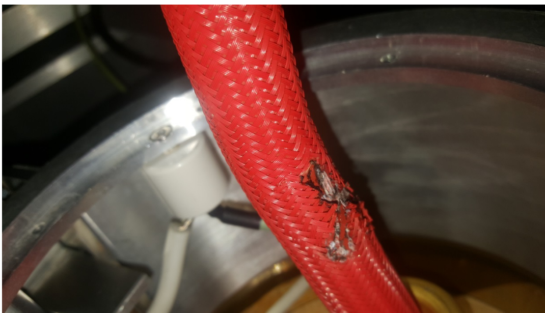
Figure 3.7: Arcing damage to the water hose
