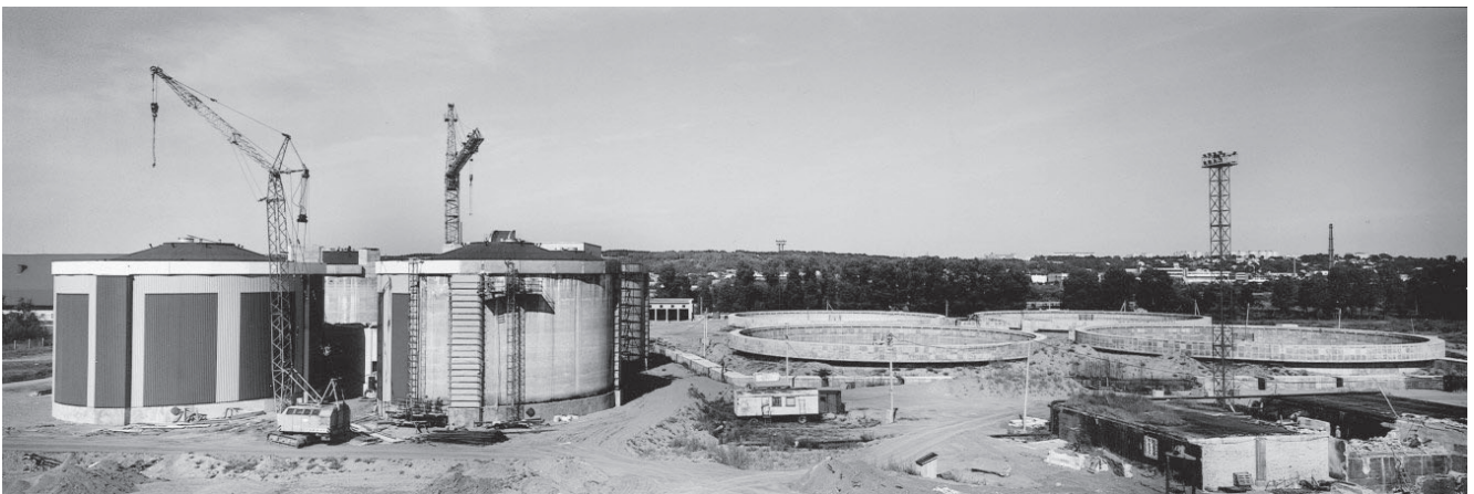
Figure 17.27. New wastewater treatment plant being built in Kaunas. Compare figure 17.10. (Source: http://www.sida.se/Sida/jsp/Crosslink.jsp?d=621&a=2896 . Photo: Courtesy Sida.)
