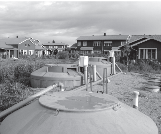
Figure 17.32. A local treatment plant in Hågaby eco-village, outside Uppsala, Sweden, receives only urine from its inhabitants. The urine is treated to be used as a perfect fertiliser on the fields close-by in cooperation with the local farmer. The households in the village all have separating water toilets, and there is a separate sewage system for urine. The black water with feces goes to the ordinary treatment plant of the city. (Photo: André Maslennikov.)
